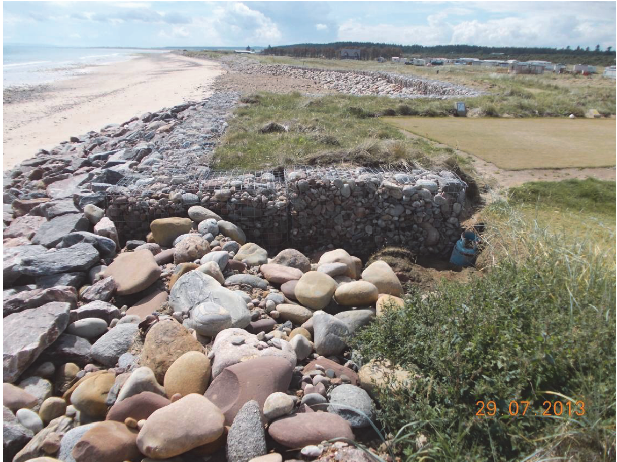
Figure 4: Position of the gabion baskets at the 7th tee and the erosional bight to the south.
