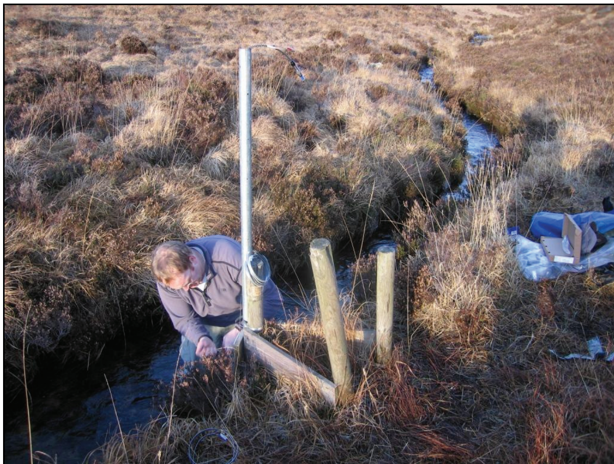
Figure 13. Installation of stilling pipe, 19 th January 2011 at the Round Loch of Glenhead outflow (Photo Chris Curtis).
