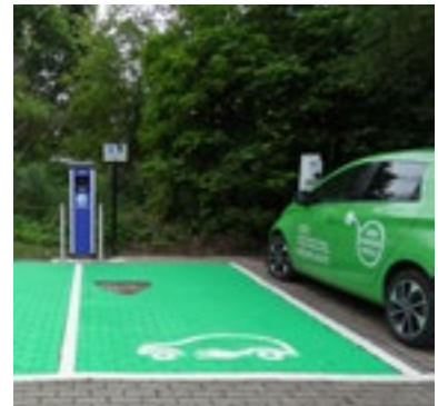
Dingwall office - dual 22kw public point.
