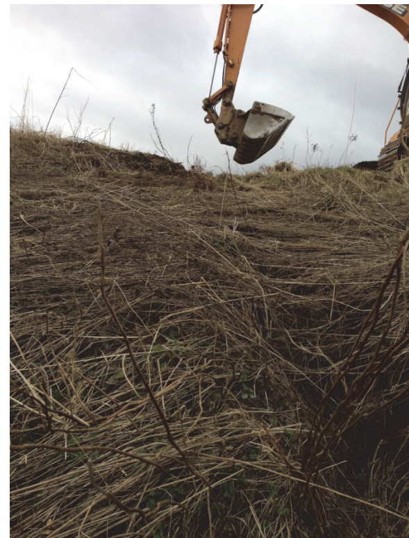
The damage from this tunnel went all the way through the flood bank.
